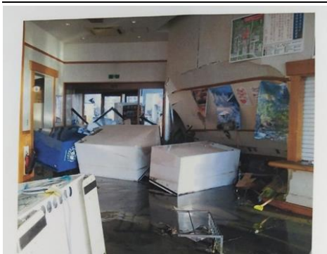
津波で自販機が流出し壁やドアを破壊(観光協会案内所窓口前) Inside the Rest House where the door and the vending machine were destroyed by the tsunami.
