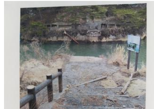
雄島に架かる「渡月橋」が津波により落下 Togetsukyo Bridge of Oshima Island washed away by the tsunami.
